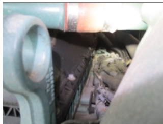
Oil, Coolant and Other Fluid Leaks
